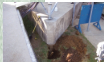
G2's Jeff Hayball, PE conducts pile integrity testing on a tower foundation
